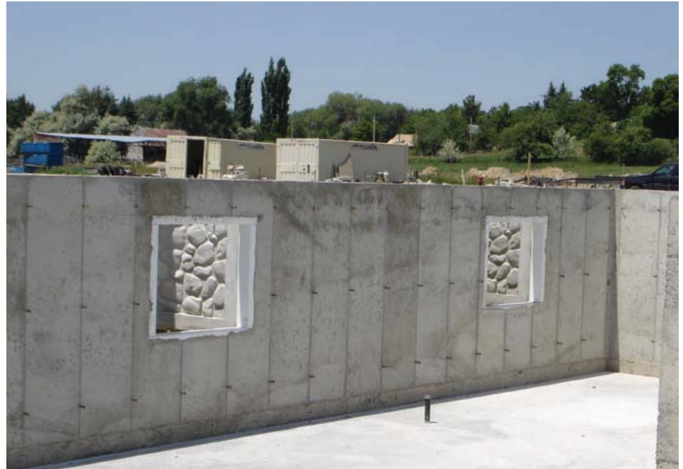
This installation of VBUCK® for poured walls in northern Utah is one of many below grade projects throughout the region.
